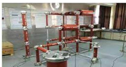
High Voltage lab
